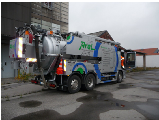
Image 14: Image: Drainage cleaning system
